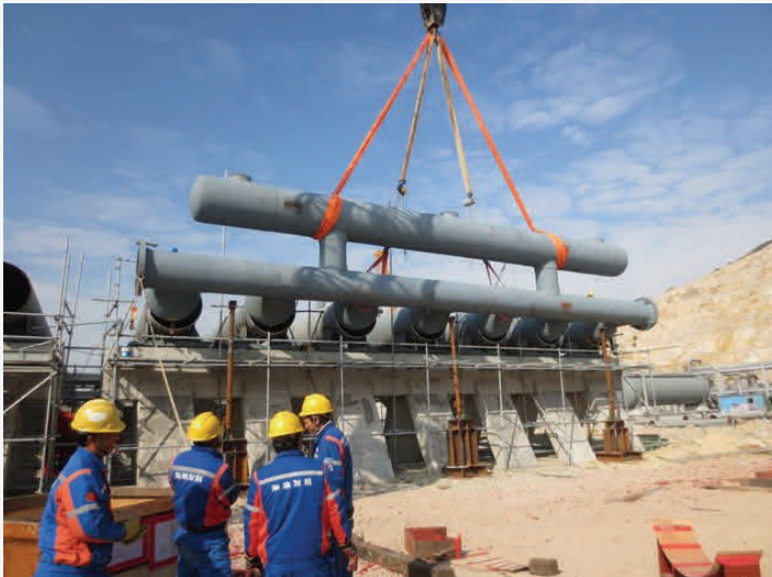
Liwan Slug Catcher Manifold Installation
